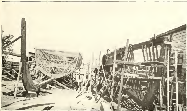
ONE HUNDRED AND TEN-FOOT SUBMARINE-CHASERS UNDER CONSTRUCTION IN A SMALL PRIVATE YARD
